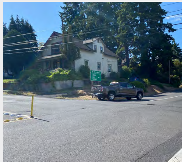
There are missing sidewalks and curb ramps at the southeast corner of May St and 13th St. Existing ramps at this intersection are considered "poor functional condition", according to ODOT's ADA inventory.
