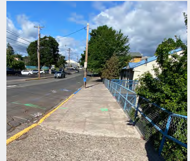
The failing elevated sidewalk at the northwest corner of 13th St and May St is slated for repairs.
